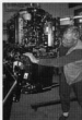
Using an engine hoist, the Merc was removed and then reinstalled with the jack plate.
